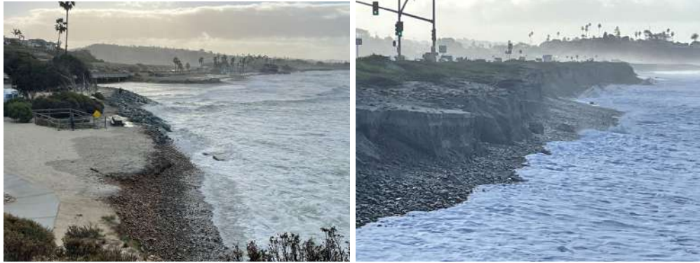
Photos 1 and 2: Erosion and storm damage of Swamis 3b and 4. Showing lack of beach access in January and February. Provided by CA State Parks.
