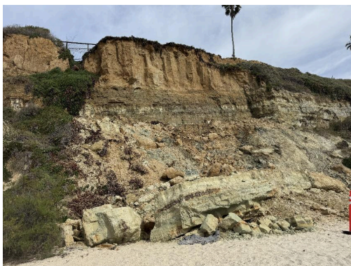
Photo 7: Block Fall at Swamis 3A in March was significant. No one was injured.
